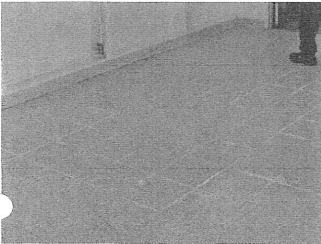
Above: Aftermath of water intrusion, winter 2011.
