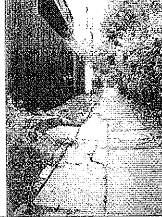
Fig. 14: Kensington's Ardmore Path (Segment 8) – Cracked pavement poses a tripping hazard and channels storm water that further degrades the pathway. Such areas need to be demolished and reconstructed.
