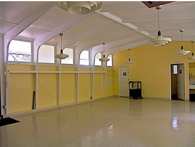
Below: Single-wall construction. Insulated stud walls could be added between the existing arches.
