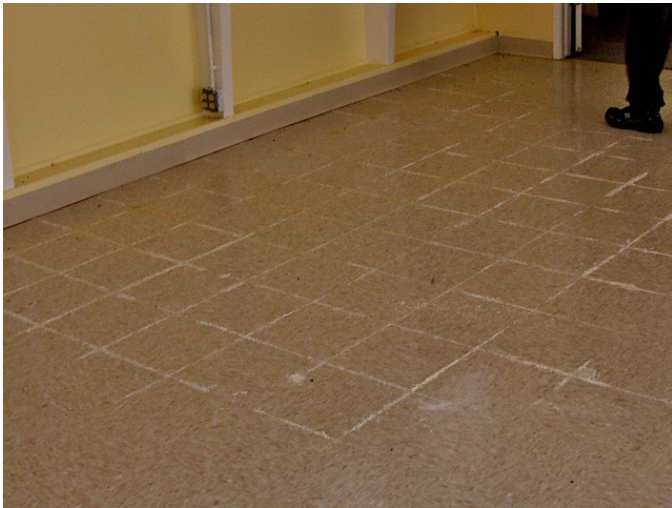
Above: Aftermath of water intrusion, winter 2011.
